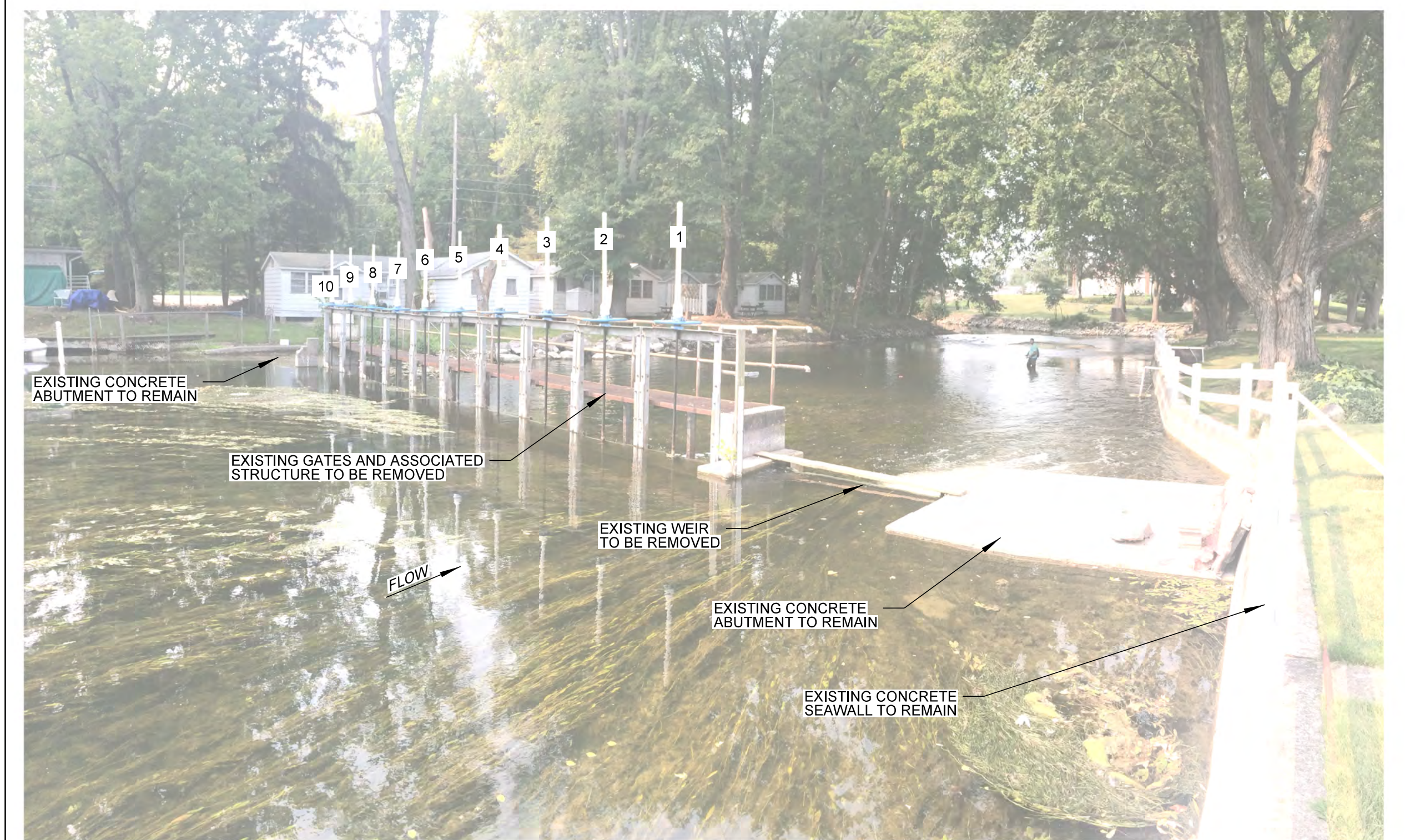
Photo taken upstream looking southwest (downstream) with Armstrong Road behind existing cabins.
