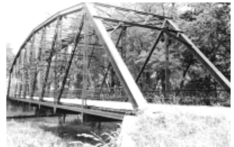
This 1916 Parker through truss was field-riveted, a tricky and unusual job for such a long truss.
