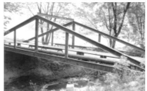
This Cantilever leg pony bridge was reinforced with a Kingpost arch, reducing the original trusses to little more than guardrails.
