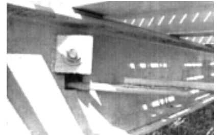
Sloppy welding repairs to this bridge make a poor substitute for proper craftsmanship.
