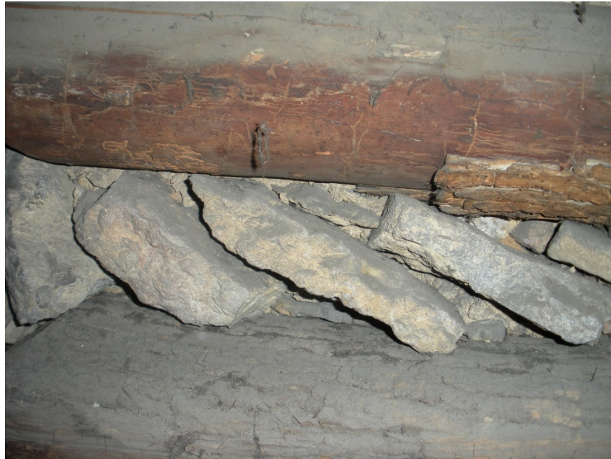
Figure 16. Anderson house stone chinking located in the roof space over the porch. Photo courtesy of Christopher Baas.
