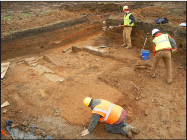
Figure 5. Crew uncovering brick foundation remnants (Features 46, 47, and 51) associated with the 1838 cell house expansion, facing northwest. (Photo credit: Kevin Cupka Head, CRA).
