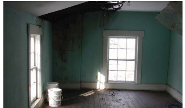
Leaking roof damage
