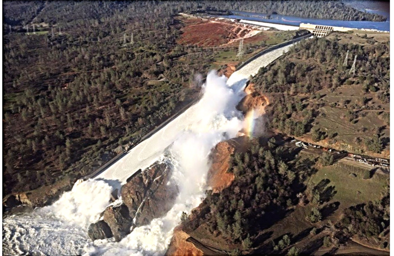
A damaged spillway with eroded hillside is seen in an aerial photo taken over the Oroville Dam in Oroville, California, U.S. February 11, 2017. California Department of Water Resources/William Croyle/Handout via Reuters
