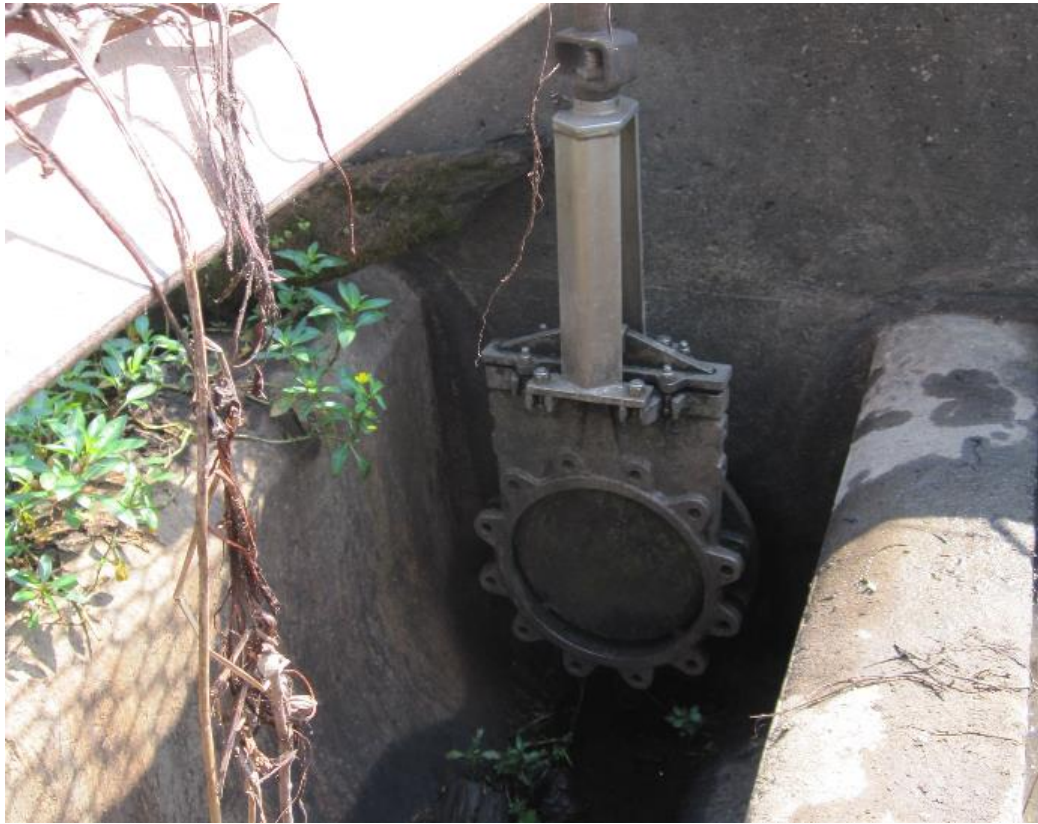
PS Riser – Drawdown Valve
