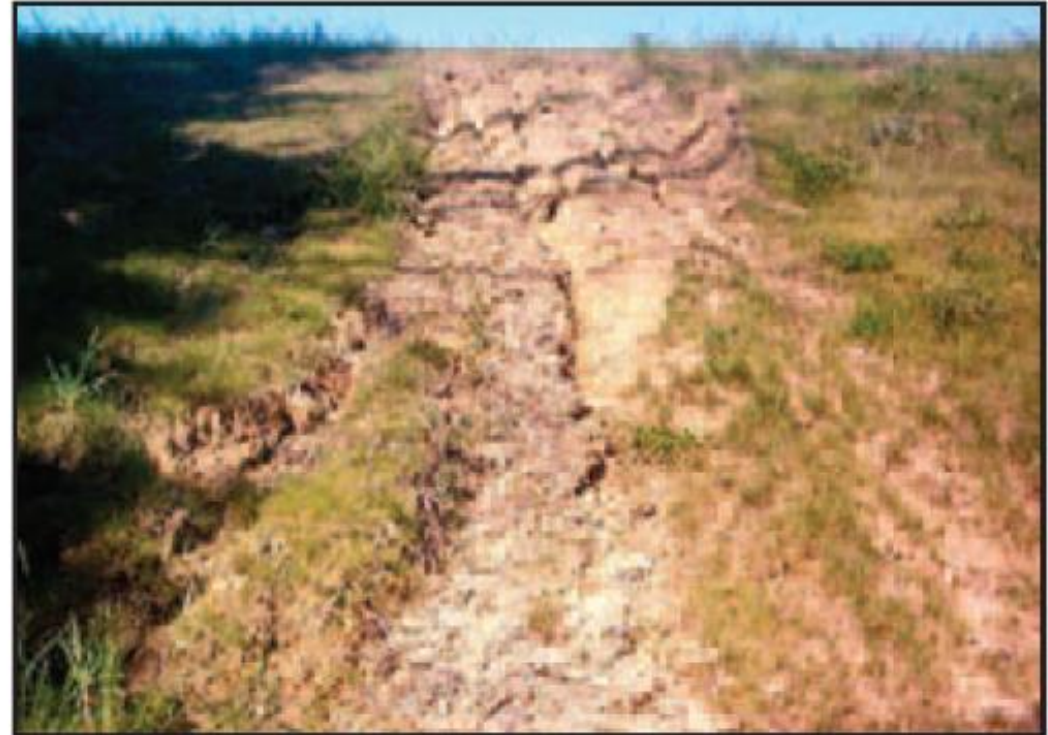
Figure 12—Erosion on the downstream face of a dam.
