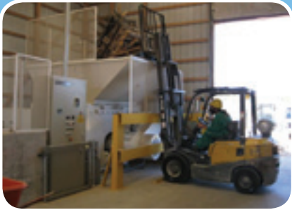
An offender operates the new wood grinder installed at Putnamville.
