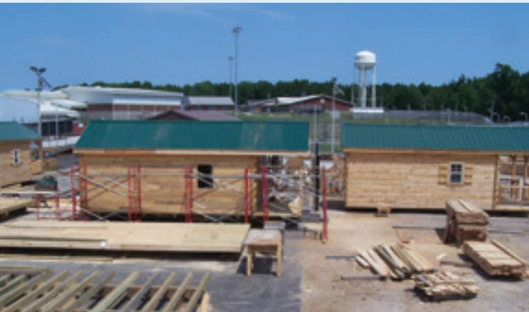
Through another partnership with DNR, staff and offenders at Branchville constructed cabins on prison grounds for use at state parks.
