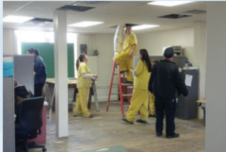
Madison Correctional Facility offenders assist with restoration of the new Madison Parole District Office.
