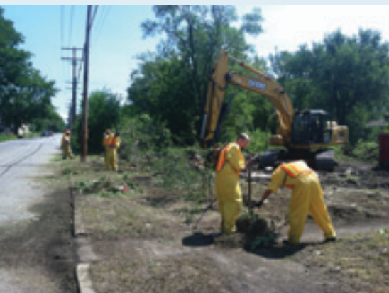
Offender work crews spent several days demolishing dilapidated houses and cleaning up parks in the City of Gary.
