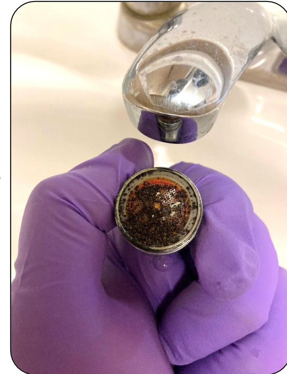
Faucet aerators should be removed and cleaned
