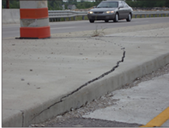
Cracks like these on the SR 62 bridge in Chandler were just part of the damage fixed by INDOT and DNR's Division of Reclamation.
