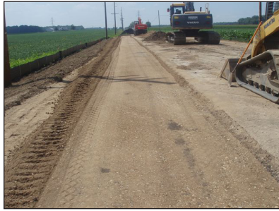
The latest project to use tire shreds as an alternative fill is pictured. This view is southbound on SR 19 in Kosciusko County.
